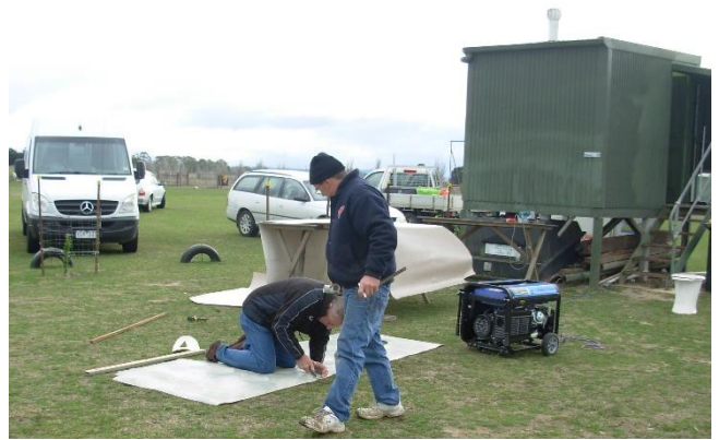
Graeme and Max (President and Vice President. Does that mean Max is in charge of the vice?) cutting the linoleum to size. What's the old saying measure twice and cut once. It's laying on the floor at the moment and looks a pretty good fit. I guess they plan to stick it down with adhesive to make sure there's no bubbles and bulges.
