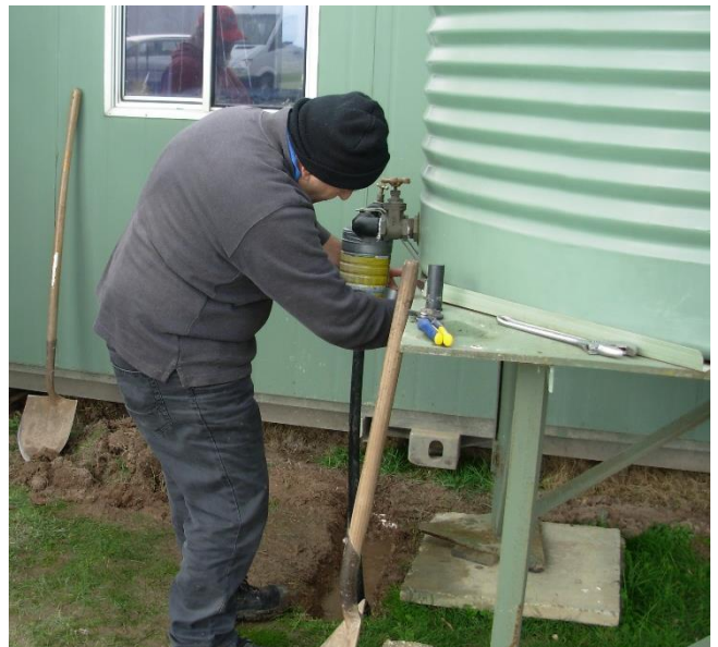
Nick turned his hand to plumbing tidying up the poly pipe from the tank to the kitchen.
